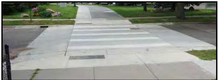
Raised Crosswalk to calm traffic
