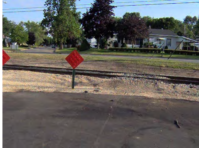
Figure 3-24: The 27 th St closure at the BNSF spur. Bicyclists have used sand and gravel to build up an area around the tracks.
