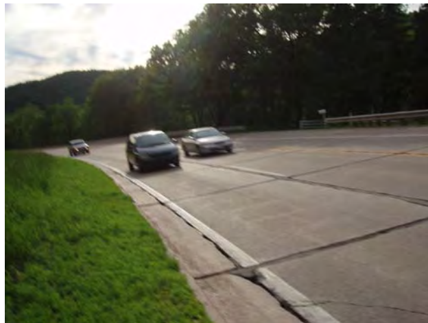
Figure 3-26: Joint cracks on STH 33. Source: Ralph Heath, bicyclist.
